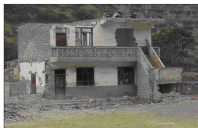
One of the collapsed primary schools that we visited.
